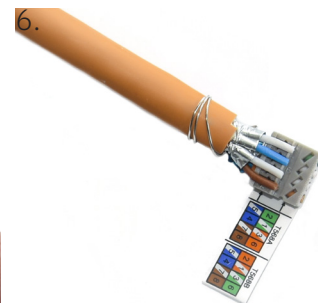
Assembled wires in the wire manager.
